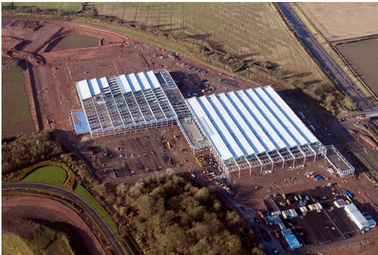
Constructing the new engine plant in the UK, with the external structure almost complete
